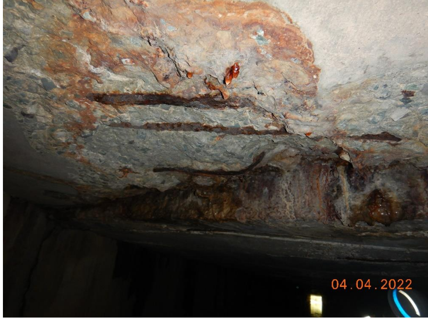
BARREL #2 - SPALL - EXPOSED REBAR - OFFSET AT CONSTRUCTION JOINT
