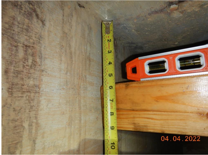
BARREL #2 - MEASUREMENT OF SAG IN THE ROOF – TAKEN AT THE INTERIOR WALL
