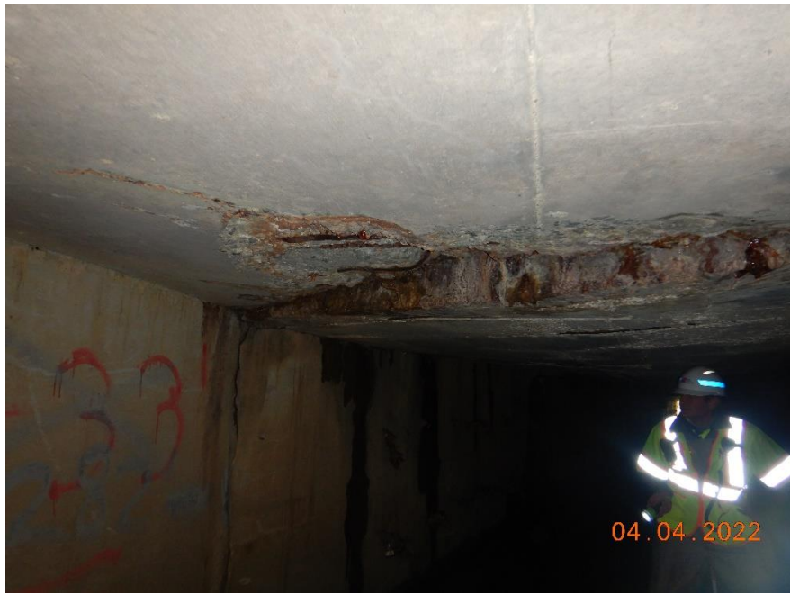
BARREL #2 - OFFSET AT CONSTRUCTION JOINT
