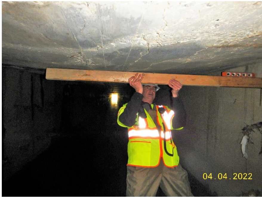
BARREL #2 - MEASUREMENT OF SAG IN THE ROOF
