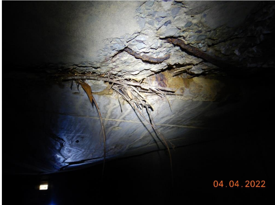
BARREL #1 - SPALL WITH EXPOSED REBAR
