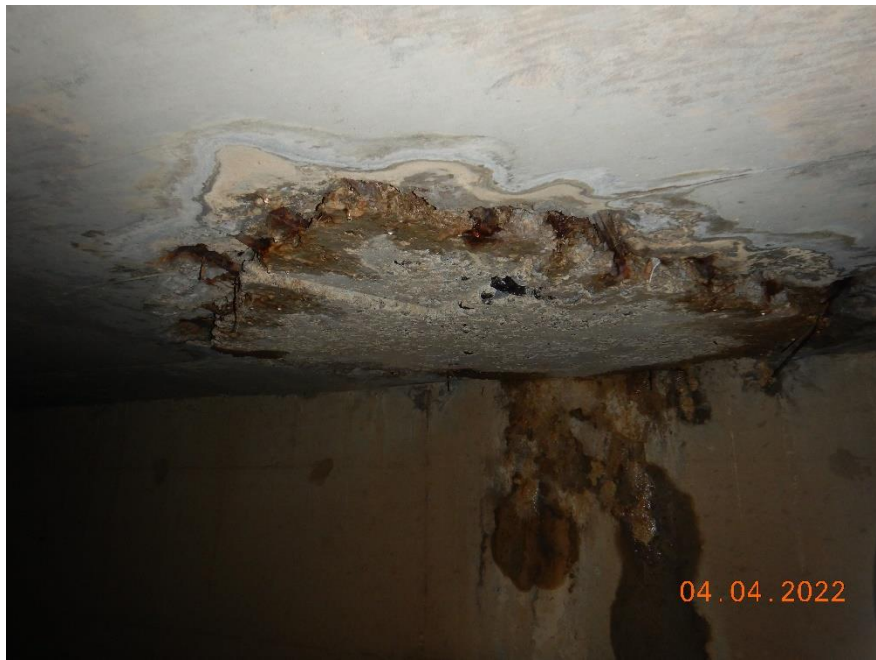
BARREL #2 - DELAMINATION-SPALL - EXPOSED REBAR – 115 FEET FROM THE INLET – 5 FEET X 5 FEET
