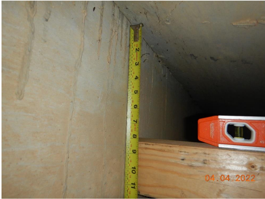
BARREL #1 - MEASUREMENT OF SAG IN THE ROOF – MEASURED AT THE EXTERIOR WALL
