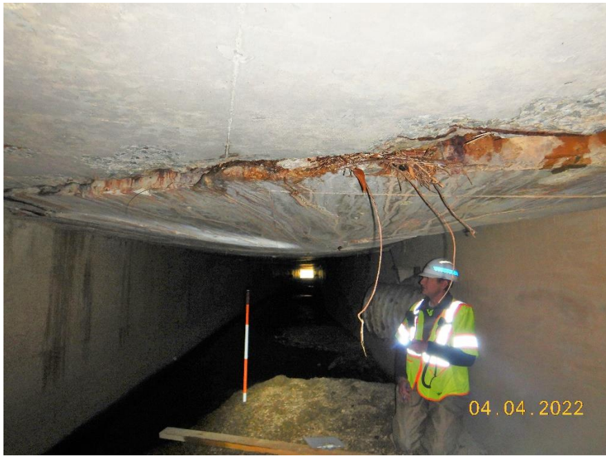
BARREL #1 - ROOF - SAG – OFFSET AT CONSTRUCTION JOINT - LOOKING TOWARD THE OUTLET
