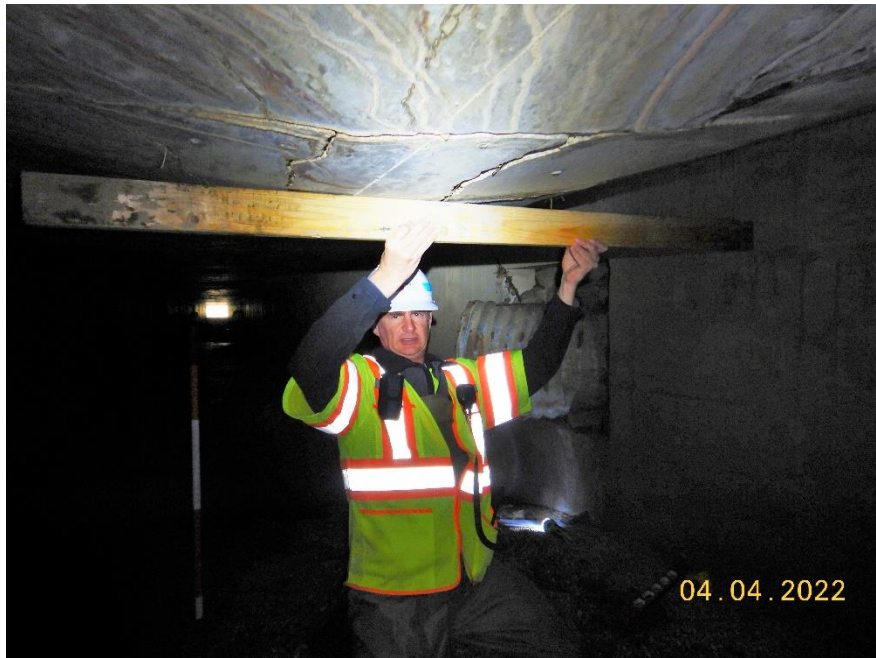
BARREL #1 - MEASUREMENT OF SAG IN THE ROOF
