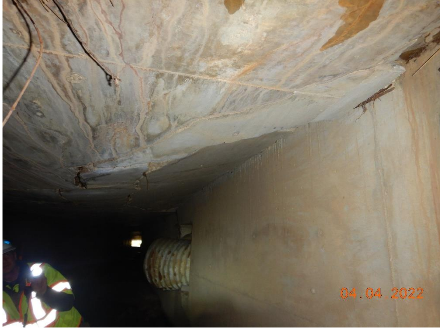
BARREL #1 - SAG IN ROOF AND DELAMINATIONS
