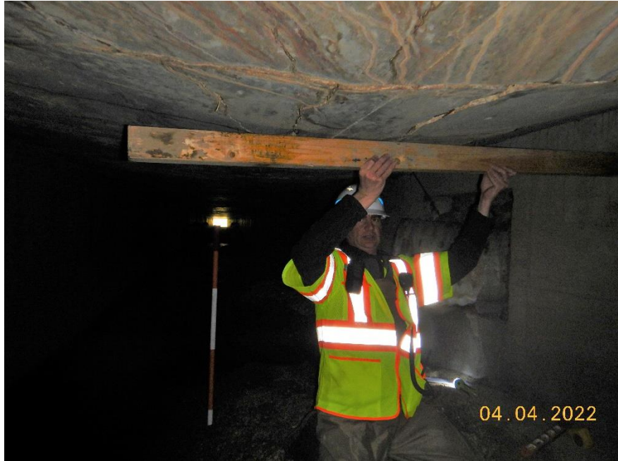
BARREL #1 - MEASUREMENT OF SAG IN THE ROOF
