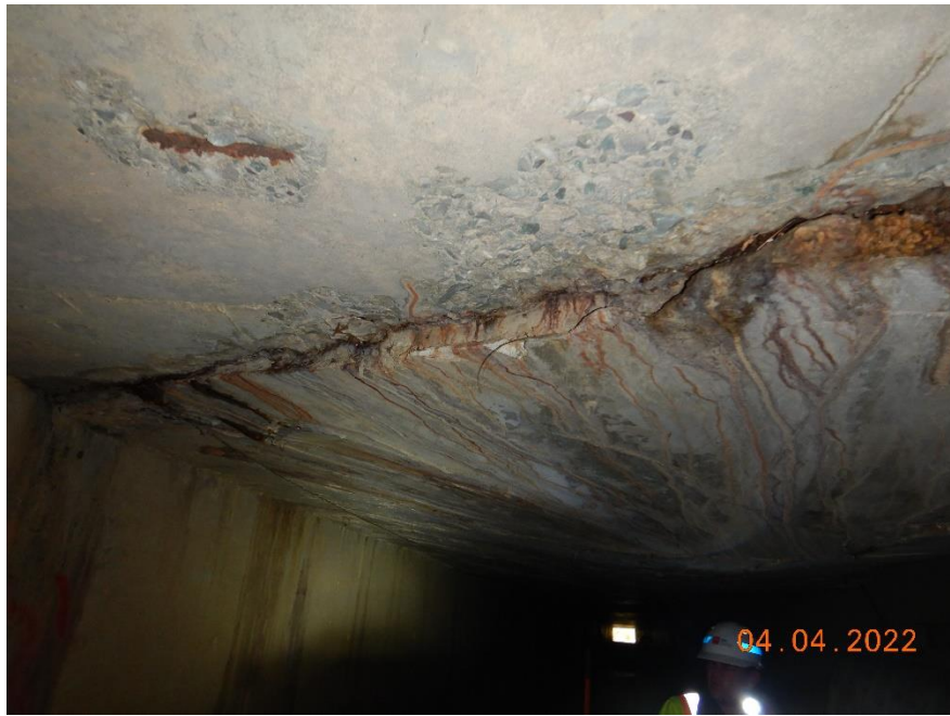
BARREL #1 - OFFSET AT THE CONSTRUCTION JOINT
