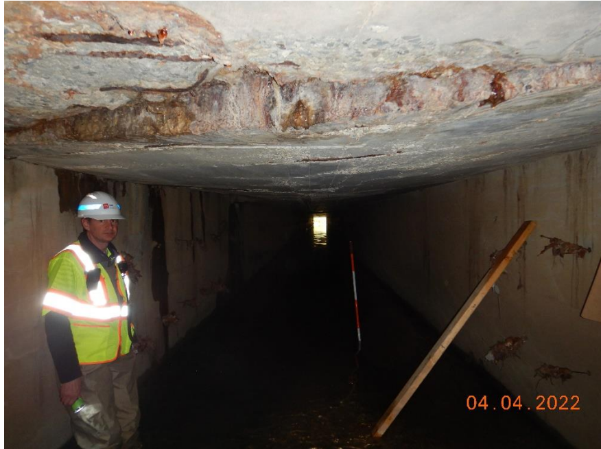
BARREL #2 - SAG IN ROOF- OFFSET AT CONSTRUCTION JOINT – LOOKING TOWARD THE OUTLET
